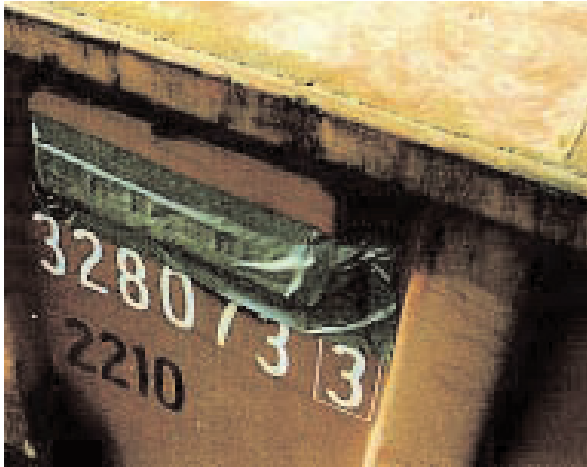
Sealed ventilation openings
