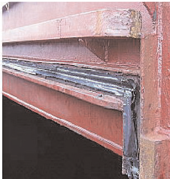
Poor practice: hatch tape used to build up cross joint. This is discouraged
