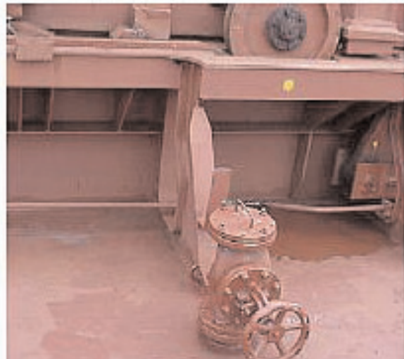
Fixed hold cleaning gun under hatch lids and fixed hold cleaning connection on deck
