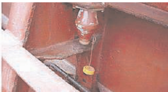
Hatch drain with cap attached by small chain
