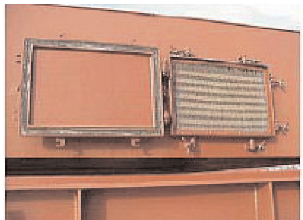
Hatch vent to secure
