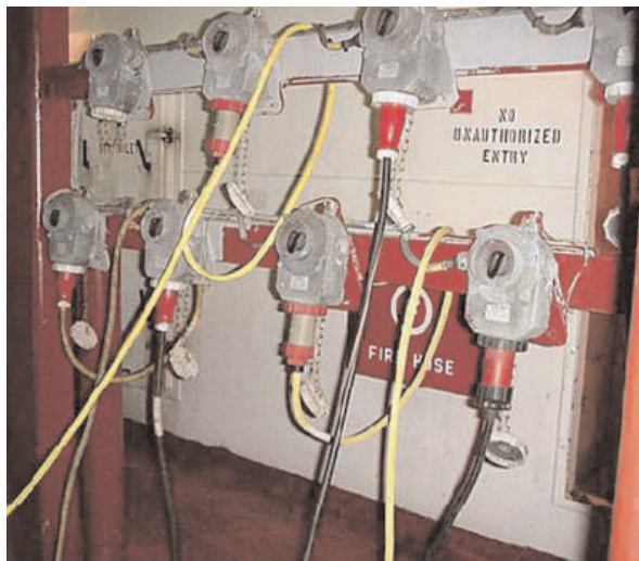
Typical sockets that connect reefer containers to the ship's power supply
