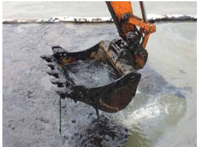
▲ Figure 21: Use of an excavator to recover highly viscous fuel oil. The concentration of recovered oil was maximised by instructing the operator to hold the bucket above the water surface for a short period, to allow entrained water to run off. This reduced the subsequent disposal costs at the expense of recovery efficiency.
