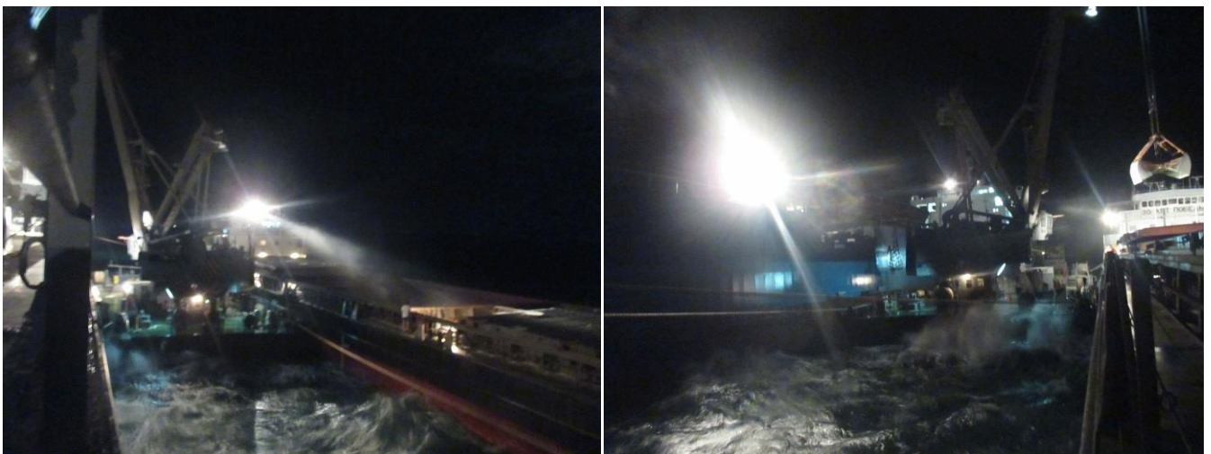
Floating crane at Kavkaz working in stormy weather, wind 14 m/sec, wave 1.5 m
