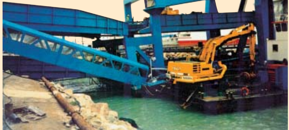
Fines totalling £1.7 million followed the collapse of this walkway
