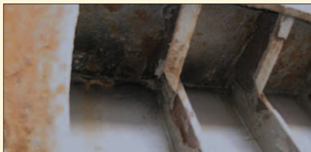
▲ 2: Corrosion of deck plating allowed phosphine gas to leak into crew cabin
