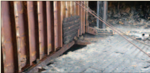
▲ View of fire-damaged tanktop sheathing, spar ceiling and burnt remains of insulation foam
