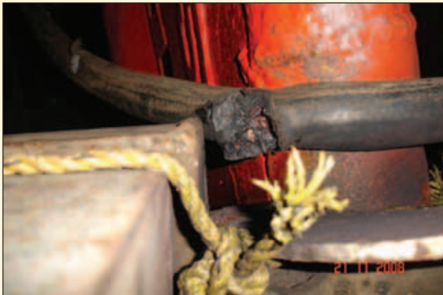
▲ Figure 5: View of the damaged power cable soon after the incident.
