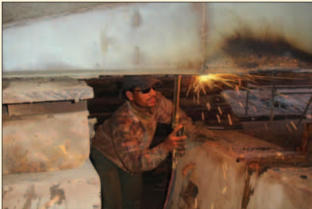
▲ Figure 3: Drydock employee wearing inadequate personal protective equipment (PPE) – right hand glove and helmet missing, eye protection does not appear to be of approved type.
