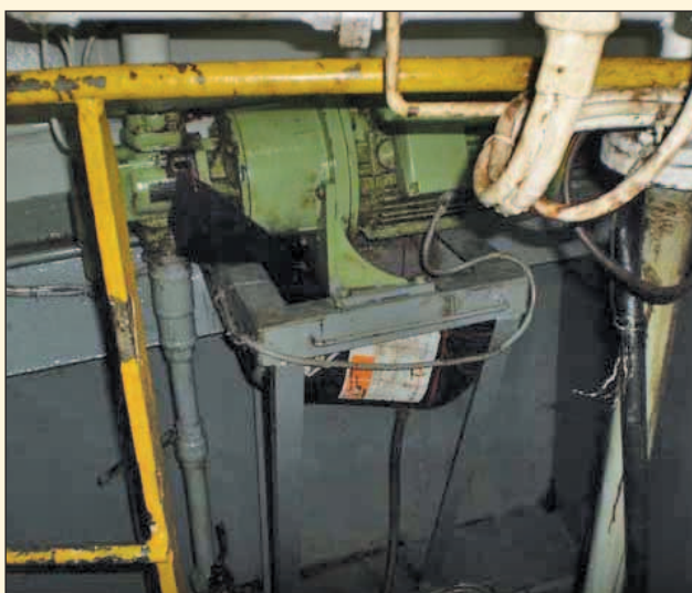
▲ Figure 3: Improvised plastic 'drip tray' fitted under sludge pump
