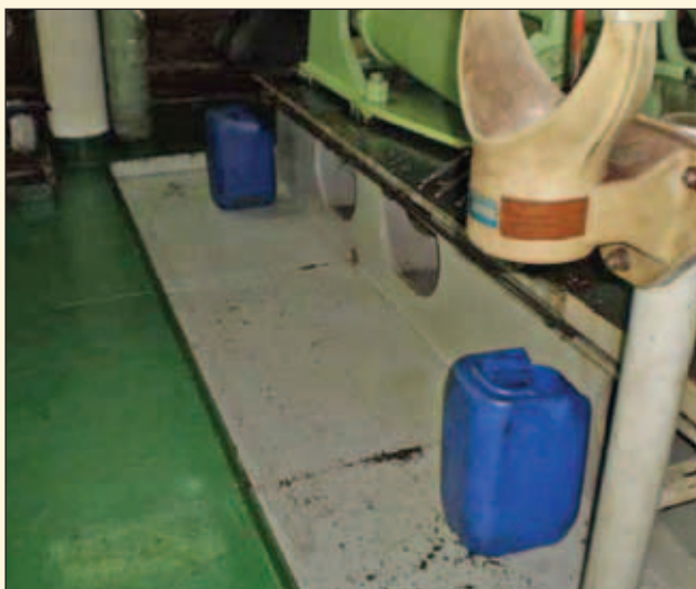
▲ Figure 4: Receptacles placed under leaking hydraulic cylinders of steering gear
