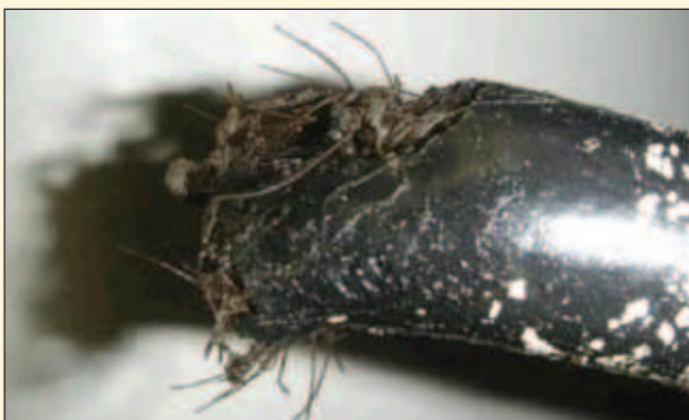
▲ Figure 2: Corroded internal wire braiding after removal of protective tape and connector
