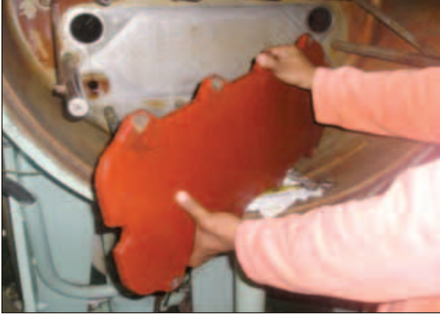
▲ Figure 1: View of FW generator cover plate coming off the holding studs
