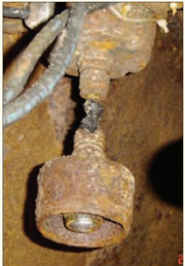
▲ Figure 3: View of the damaged light fixture with exposed live components
