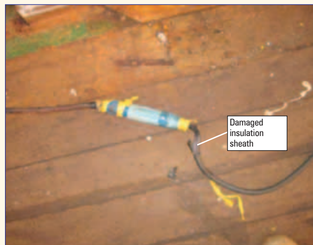
▲ Figure 4: Damaged insulation sheath
