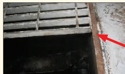
◀ Figure 3: View of loose and under-size grating
