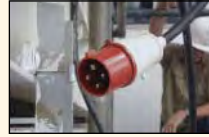
▲ Unsafe live male plug with exposed conductors
