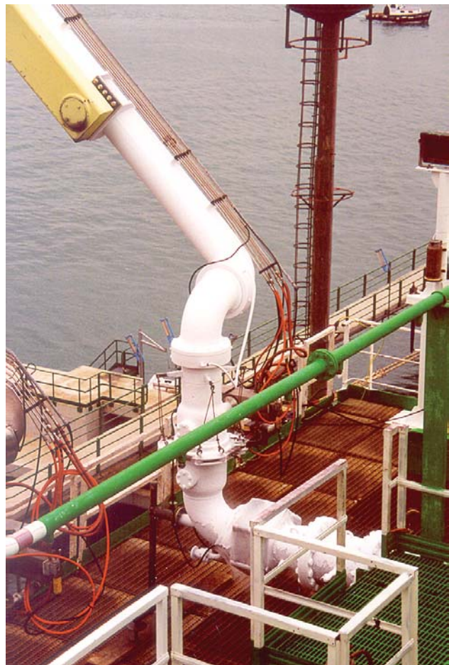
Hard arm connection to manifold, showing double ball valve safety release
