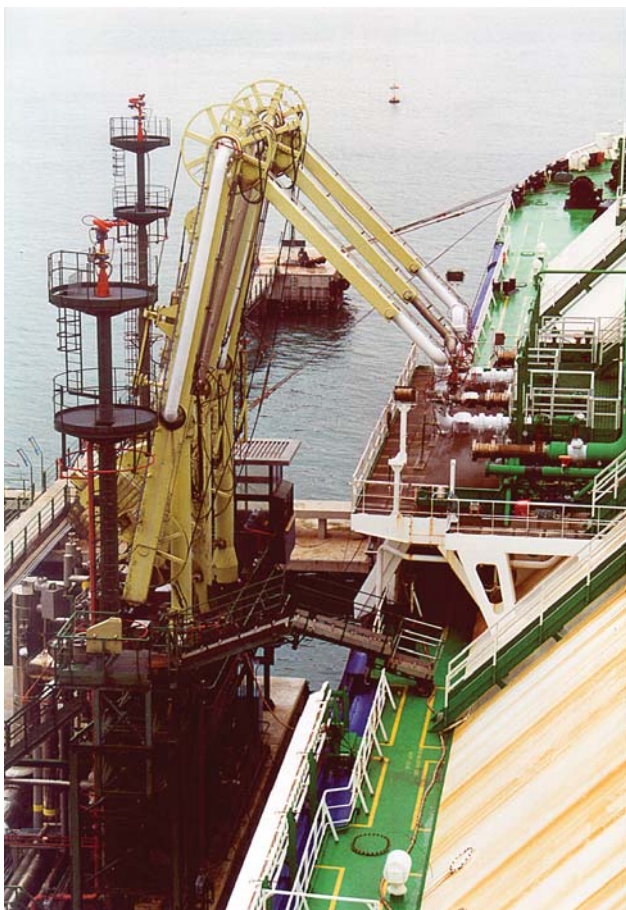
Hard arms at cargo manifold, including vapour return line
