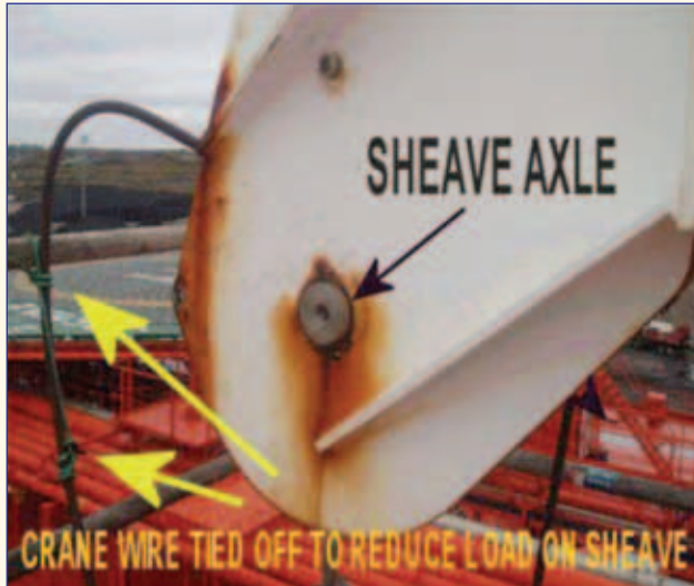
▲ Figure 4: Crane wire tied off to reduce load on sheave
