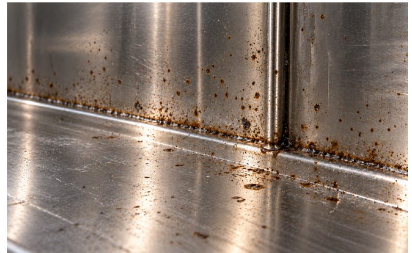
Example of pitting corrosion.
