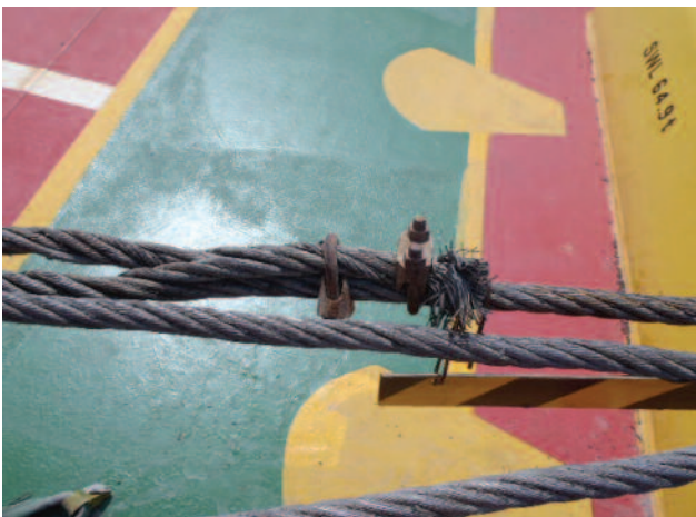
Insufficient number of staggered grips, too close together and wire tail too short
