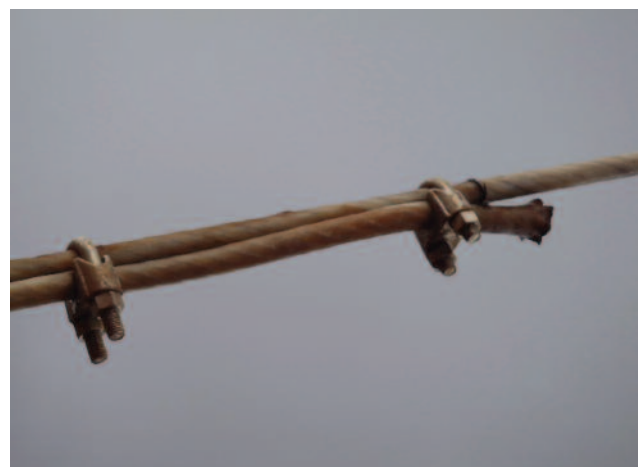
Too few bulldog grips reversely applied over a plastic coating and too far apart
