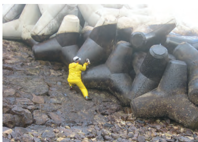
▲ Figure 33: Cleaning of oiled tetrapods is problematic, as oil within the structure is difficult to reach.
