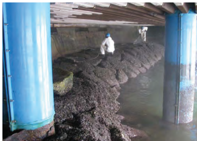
▲ Figure 31: Access underneath wharves may be difficult and dangerous for clean-up crews due to the lack of headroom and ventilation.
