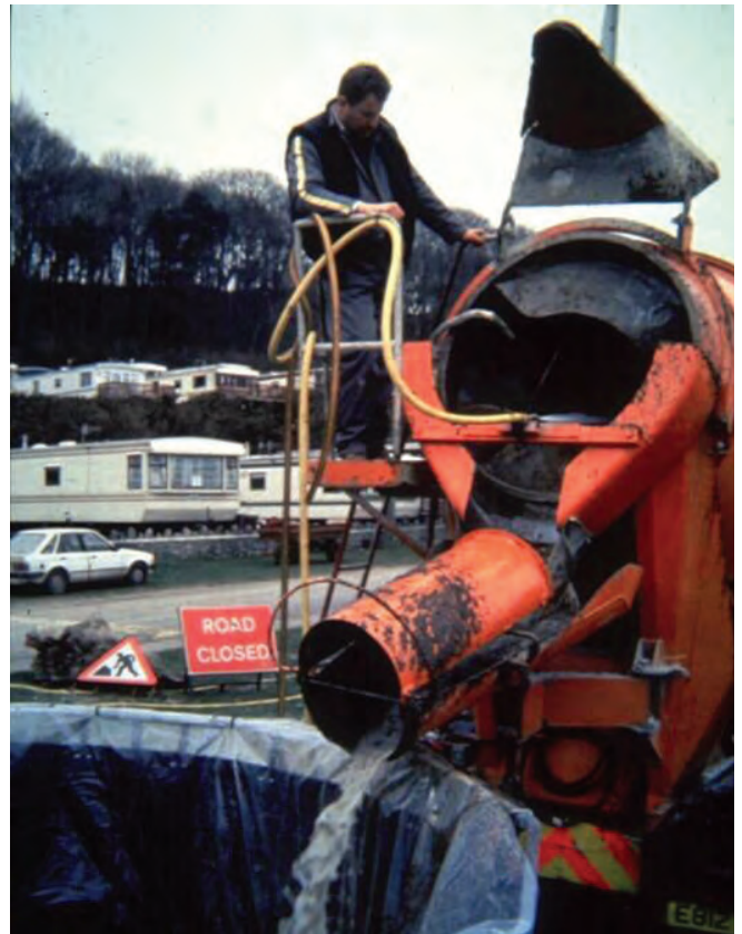
▲ Figure 24: Effluent released from a concrete mixer truck after washing pebbles and small cobbles.
