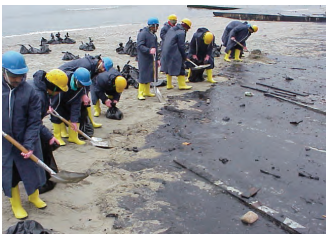
▲ Figure 9: An area of stranded fuel oil manually collected using shovels and placed into bags.
