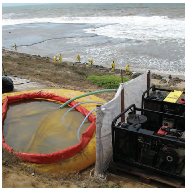
▲ Figure 22: Pressure cleaning a rock ledge in a remote location. Seawater was pumped to the temporary storage tank to be used by the adjacent high pressure machines.
