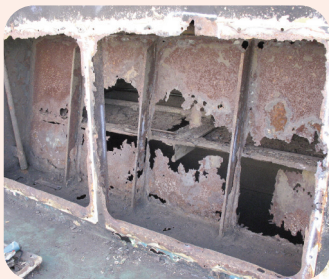
Fire damper wastage found after removing cover.
