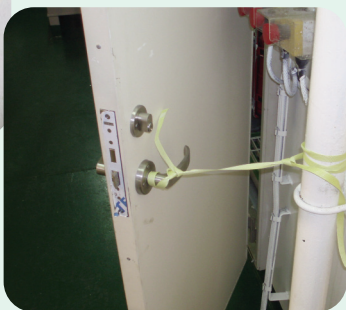
Fire door held open using an unapproved method.
