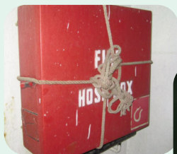
Fire hose box tied shut using an unapproved method.
