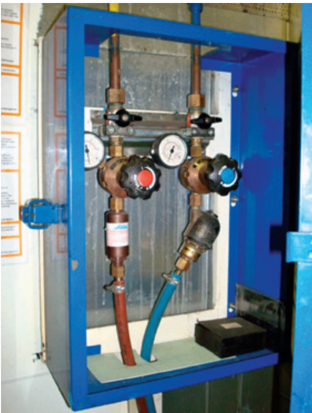
Interior of good welding cabinet in Engine Room workshop
