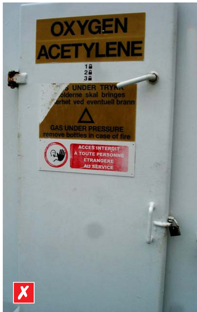
Bad stowage – mixed cylinders in enclosed locker
