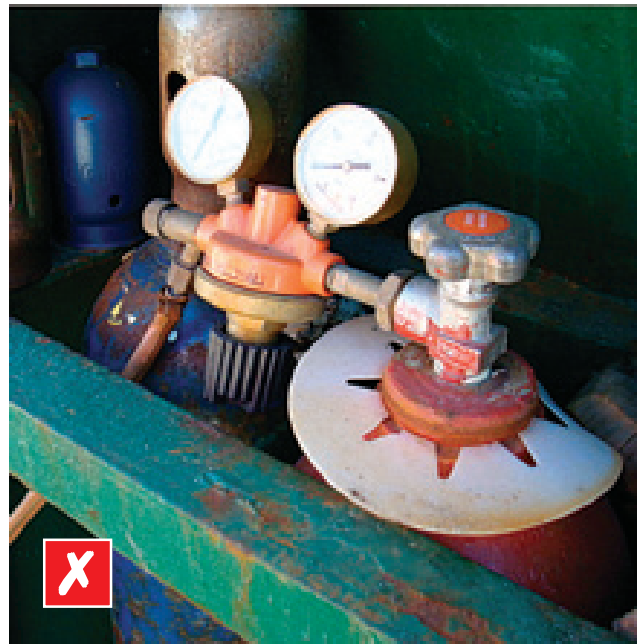
No flash back arrestor fitted, and poor stowage could lead to explosion
