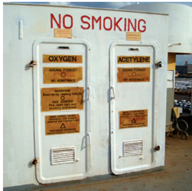
Good stowage – segregated and well marked lockers on deck.
