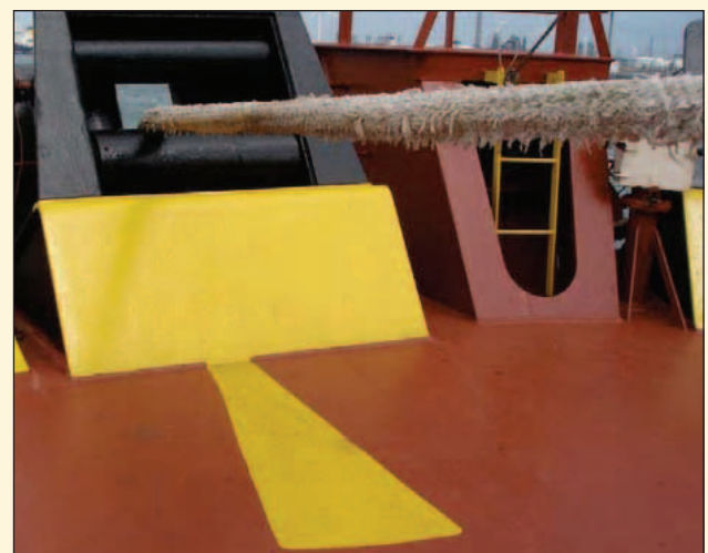
▲ Figure 4: Snap-back zone marked in way of a single multi-angle roller fairlead
