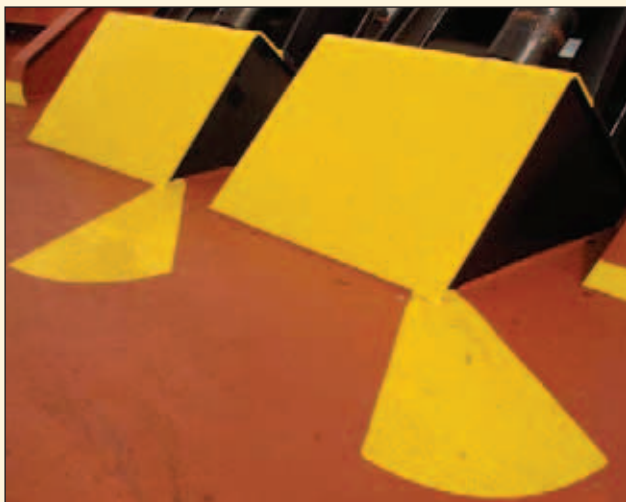
▲ Figure 5: Snap-back zones marked in way of a double multi-angle roller fairlead
