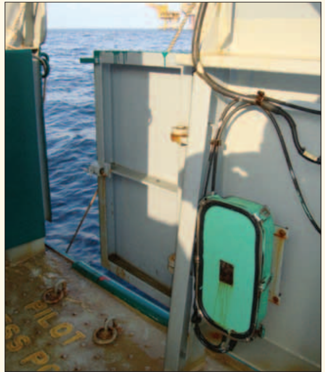
▲ Figure 8: Electrical junction box in a location frequently subject to sea water inundation. On this ship, all the circuits fed from this box were damaged.
