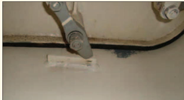
▲ Figure 4: Watertight escape hatch with wedge welded in wrong orientation
