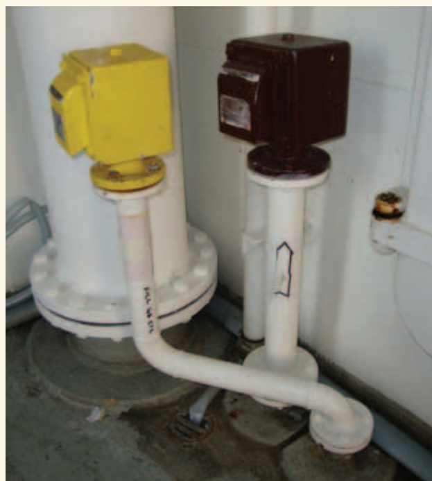
▲ Figure 6: Oil tank vents without a save-all and located directly over an open deck scupper. The marking seems to suggest that the crew is using the vent line for filling the tank, which increases the risk of spills.
