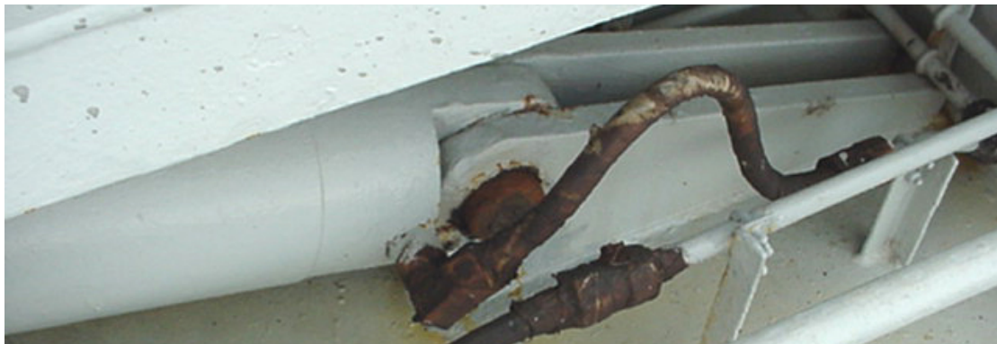
Hatch cover hydraulics (this image is not associated with any of the incidents described in this bulletin)
