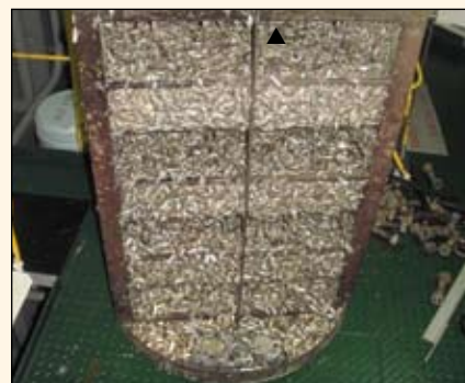
◀ View of clogged strainer of sea chest
