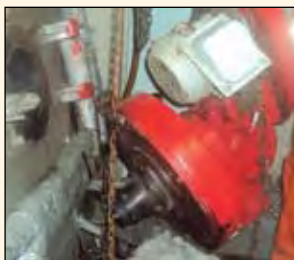
▲ Burner assembly removed and atomizer holes found blocked by unburnt residue and debris
