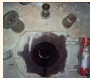
▲ View of burner assembly port showing evidence of oil accumulation
