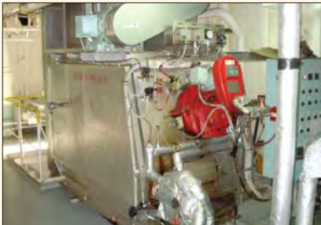
▲ Exterior view of incinerator
