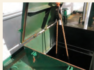
Improperly secured open lid wrongly being used to lift loads
