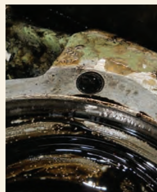
Close-up view showing sheared bolt of filter cover
