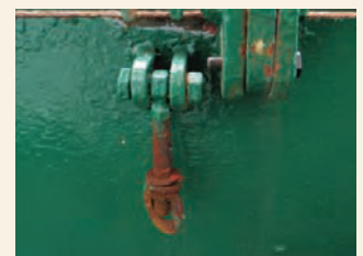
Non-standard bolt was used in place of a safer 'drop-nose' pin
