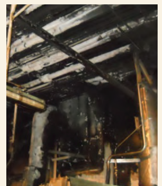
View of fire damage
