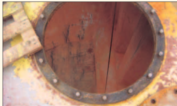
▲ Figure 3: View of unsafe deck opening
