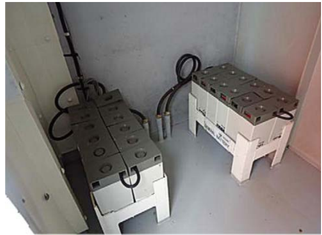
The battery room to be maintained in clean state
