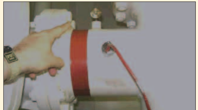
▲ Close-up view showing redundant probe connector with isolating cock and second probe connector in use.
