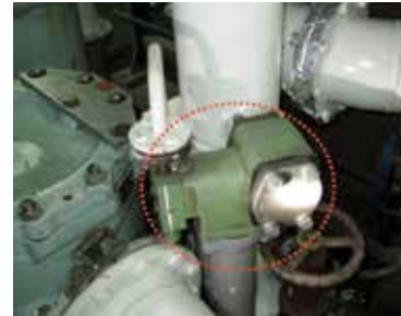
Pressure control valve as installed
